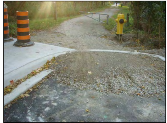
Construction near David Street—temporary conditions are hazardous for cyclists on the Iron Horse Trail
