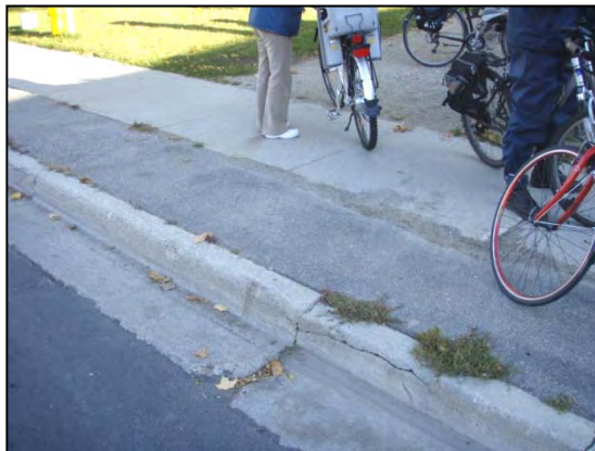
No curb cut on Krug Street at “Becker Street” Community Trail
