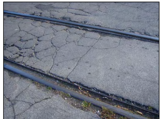
Wellington Street rail crossing—rough tracks
