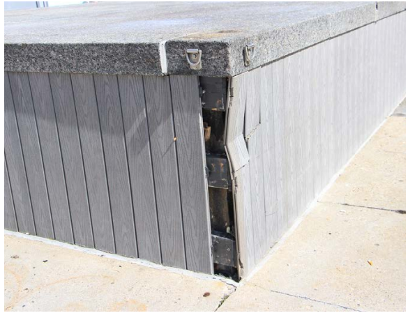
Fig. 32 Missing and broken siding along the edge of the stage.
