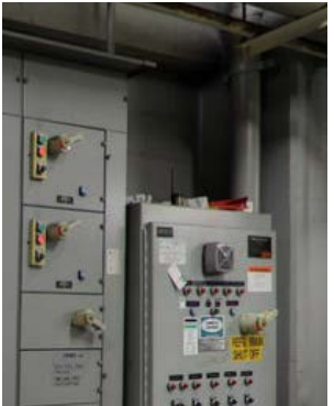
Fig. 31 Existing electrical equipment for the fountain is still in good condition after 20+ years of use.
