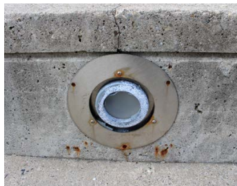
Fig. 36 Wall lights are starting to show signs of wear due to heavy salting of the civic spaces during the winter months.
