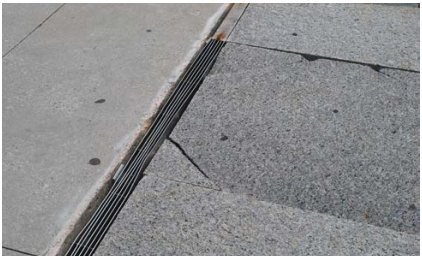
Fig. 28 Example of cracked granite paving along the edge of an existing trench drain.
