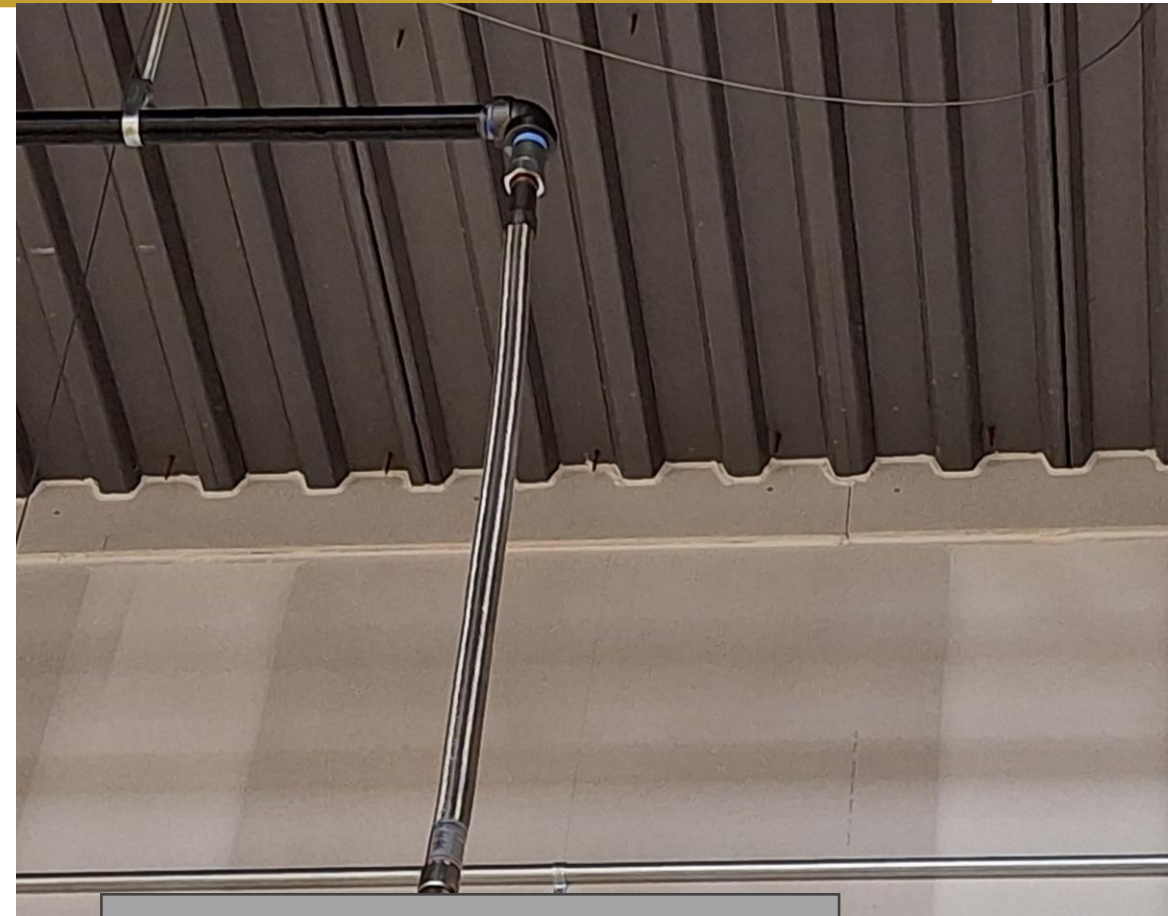
Firestopping of joint where fire rated wall abuts unrated roof
