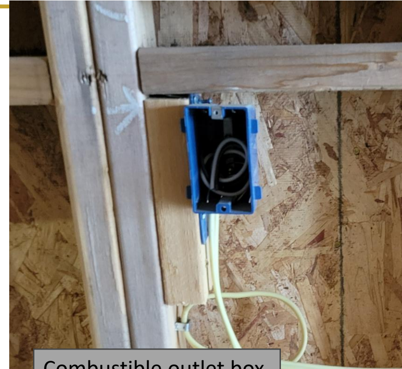
Combustible outlet box requires firestop
