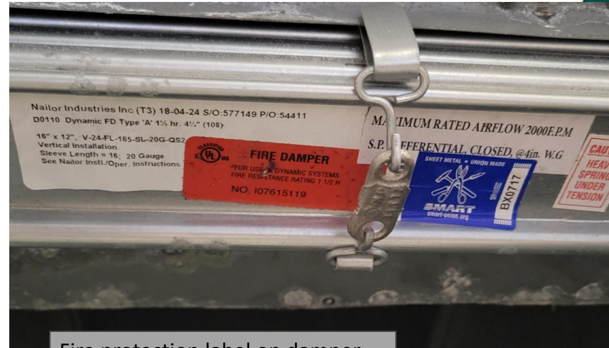
Fire protection label on damper
