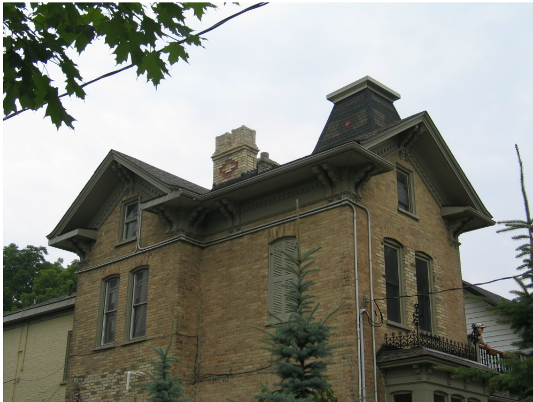
31 Margaret Avenue -decorative brick chimney missing top courses
