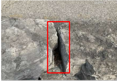
#28 - Area 2 - Monitor adjacent boulders as large gaps are present that pose foot entrapment hazards
