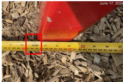
#19 - Area 3 - Protective surfacing zone is short on one (1) side of Saucer Swing Set (measures ~ 1.5m)
