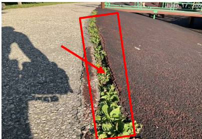
#5 - Area 1 - Rubber surfacing is damaged (torn, loose, missing), receding from asphalt, and lifting from asphalt in spots
