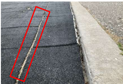
#13 - Fitness Area - Rubber tile surfacing is uneven (heaved and sunk) and separated in spots
