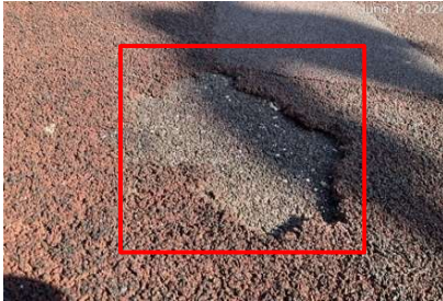
#10 - Area 1 - Rubber surfacing is damaged (torn, loose, missing), receding from asphalt, and lifting from asphalt in spots
