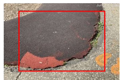
#9 - Area 1 - Rubber surfacing is damaged (torn, loose, missing), receding from asphalt, and lifting from asphalt in spots
