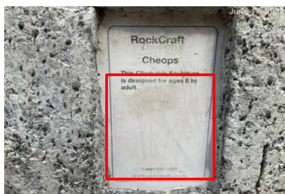
#25 - Area 2 - Label at Boulder Climber is worn and missing info (not legible)
