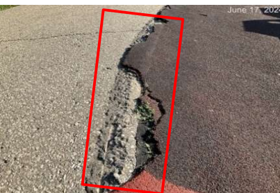
#8 - Area 1 - Rubber surfacing is damaged (torn, loose, missing), receding from asphalt, and lifting from asphalt in spots
