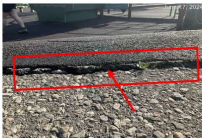
#7 - Area 1 - Rubber surfacing is damaged (torn, loose, missing), receding from asphalt, and lifting from asphalt in spots
