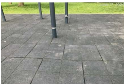
#16 - Fitness Area - Rubber tile surfacing is uneven (heaved and sunk) and separated in spots
