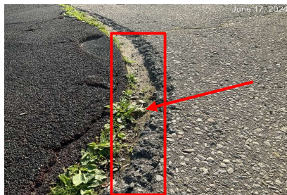
#4 - Area 1 - Rubber surfacing is damaged (torn, loose, missing), receding from asphalt, and lifting from asphalt in spots
