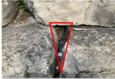
#29 - Area 2 - Monitor adjacent boulders as large gaps are present that pose foot entrapment hazards
