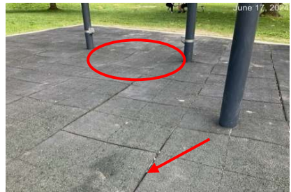
#15 - Fitness Area - Rubber tile surfacing is uneven (heaved and sunk) and separated in spots
