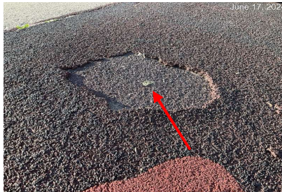
#2 - Area 1 - Rubber surfacing is damaged (torn, loose, missing), receding from asphalt, and lifting from asphalt in spots
