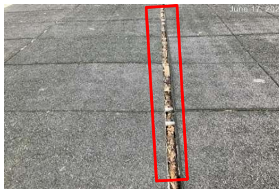
#14 - Fitness Area - Rubber tile surfacing is uneven (heaved and sunk) and separated in spots
