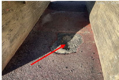
#1 - Area 1 - Rubber surfacing is damaged (torn, loose, missing), receding from asphalt, and lifting from asphalt in spots
