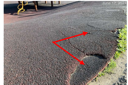
#3 - Area 1 - Rubber surfacing is damaged (torn, loose, missing), receding from asphalt, and lifting from asphalt in spots
