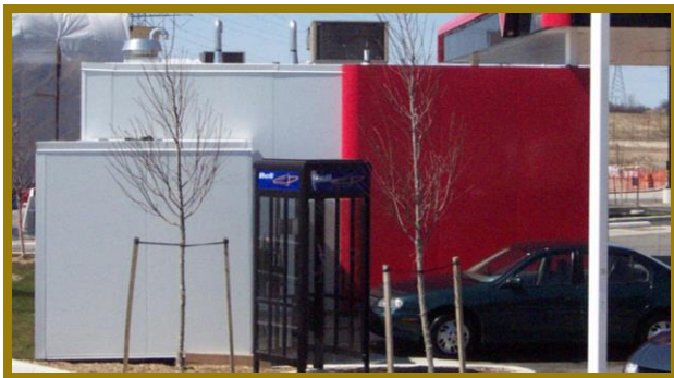
Figure 7.7: The rooftop equipment on this corner gas station is not screened and is visible from public view.
